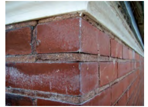
Some tuck pointing needed
