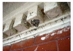
Failing paint on dentil detail
