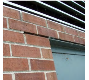
Failed mortar joints
