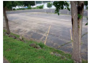
Parking lot needs repair
