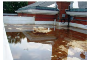
Standing water on roof due to obstructed drains
